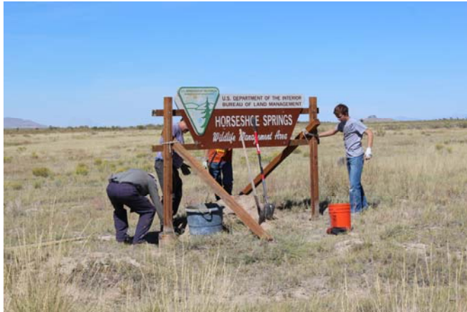
Installing interpretive wayside exhibits and site signs on a National Public Lands Day project at Horseshoe Springs in Skull Valley, Utah – September 30, 2013.
